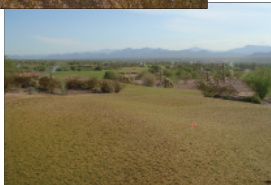
We-Ko-Pa Golf Club, Saguaro, AZ. Course hole. No. 10 Top: Construction. Bottom: Hydroseeding
